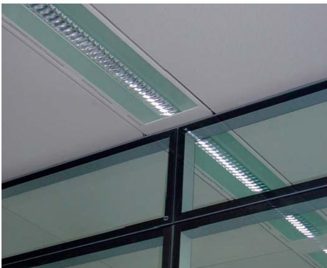
Fig. 60 Metal ceiling with recessed light fixture and fully glazed partition
